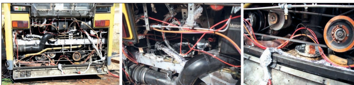
Fig. 44: Engine compartment equipped with fire detection and fire suppression systems
