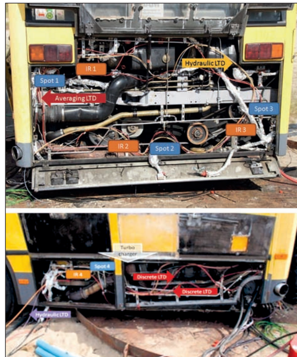
Fig. 45: Tested fire detection systems and their locations in the engine compartment
