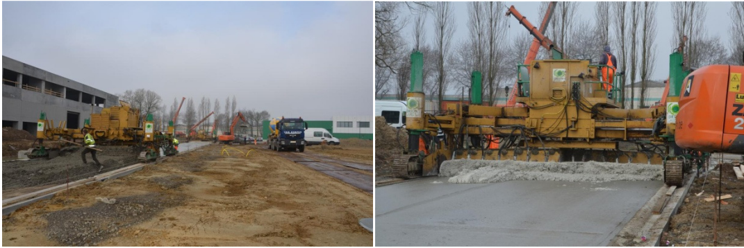
Figure 7 – Construction of the double layered concrete pavement at “Den Hoek 3” in Wijnegem.
