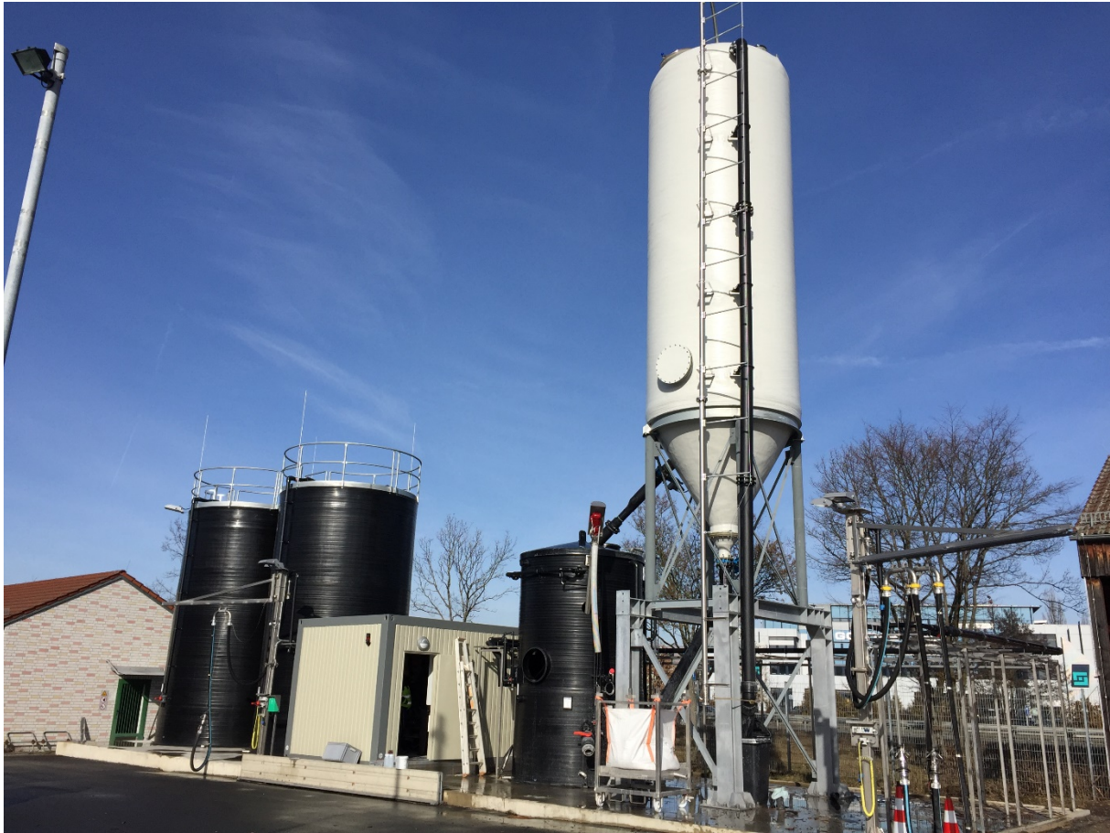
Continuously working brine production system with salt silo, technology container and brine tanks in the AM Erlangen (Picture: Salt Research & Consulting)
