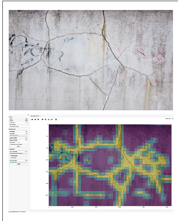
Fig 2: Example of a crack-damaged concrete surface with disturbances in the image (top), result (heat map) of the automatic image analysis with the developed software tool (bottom)
