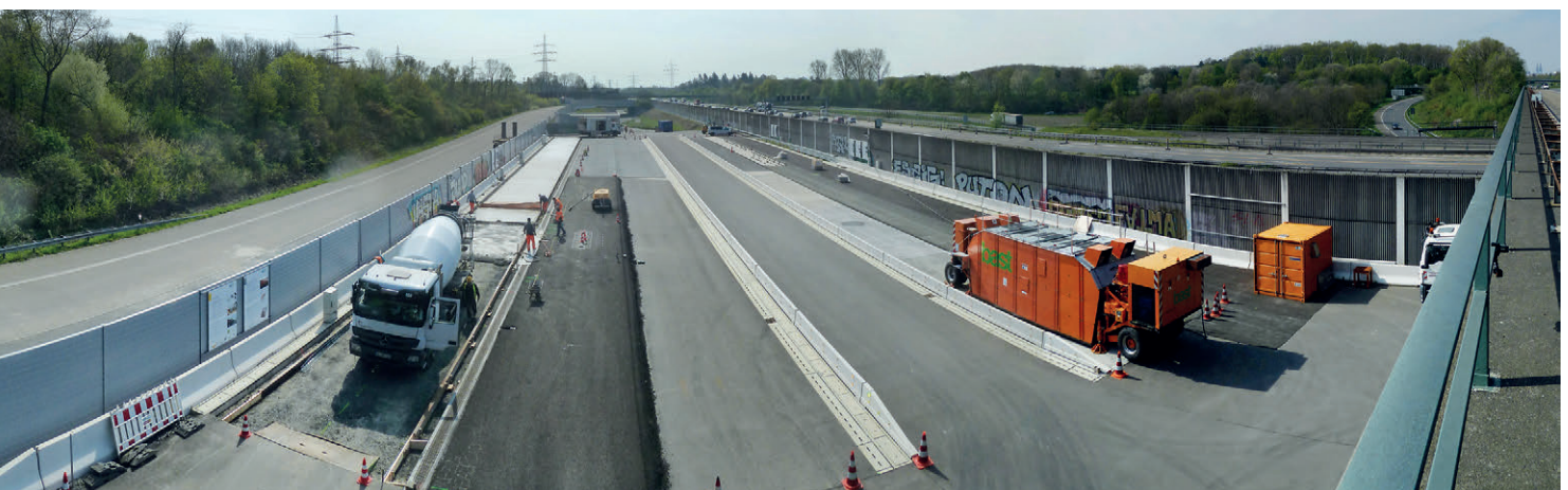
Installing a concrete carriageway on duraBAST (left) – on the right the Mobile Load Simulator MLS30
