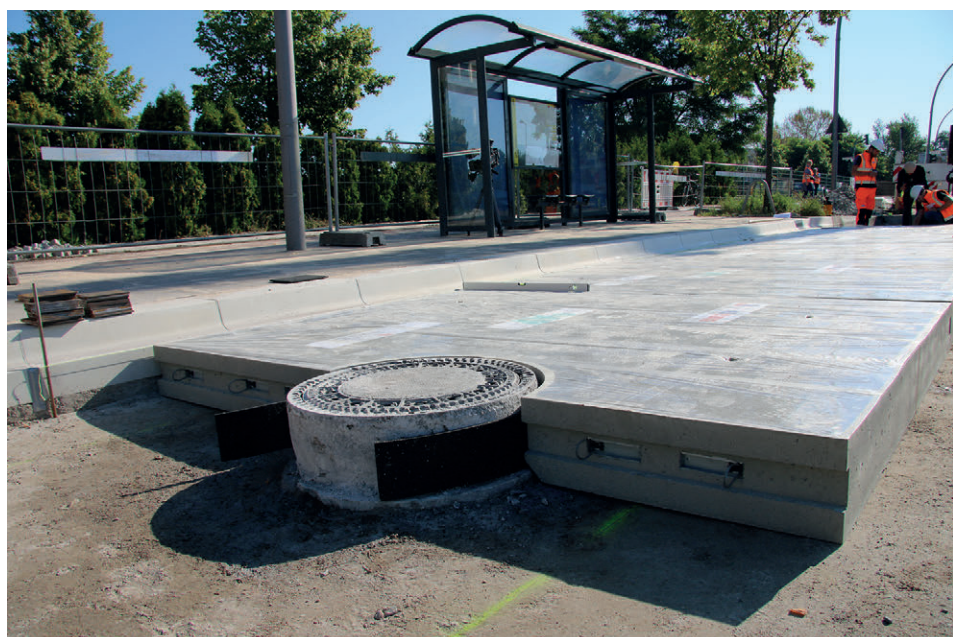
Prefabricated element with recess around manhole structure after installation and height adjustment
