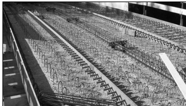
Figure 2: Headed studs close to the concrete edge in cross section at a bridge over the main road B465 at Münsingen
