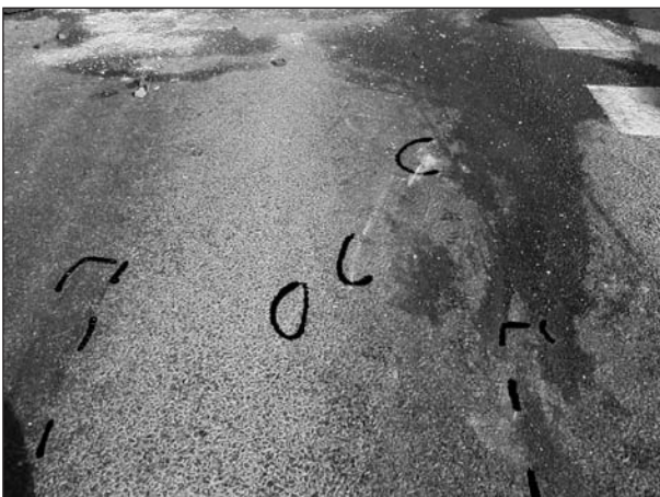
Fig. 6: Scratching marks, point of impact
