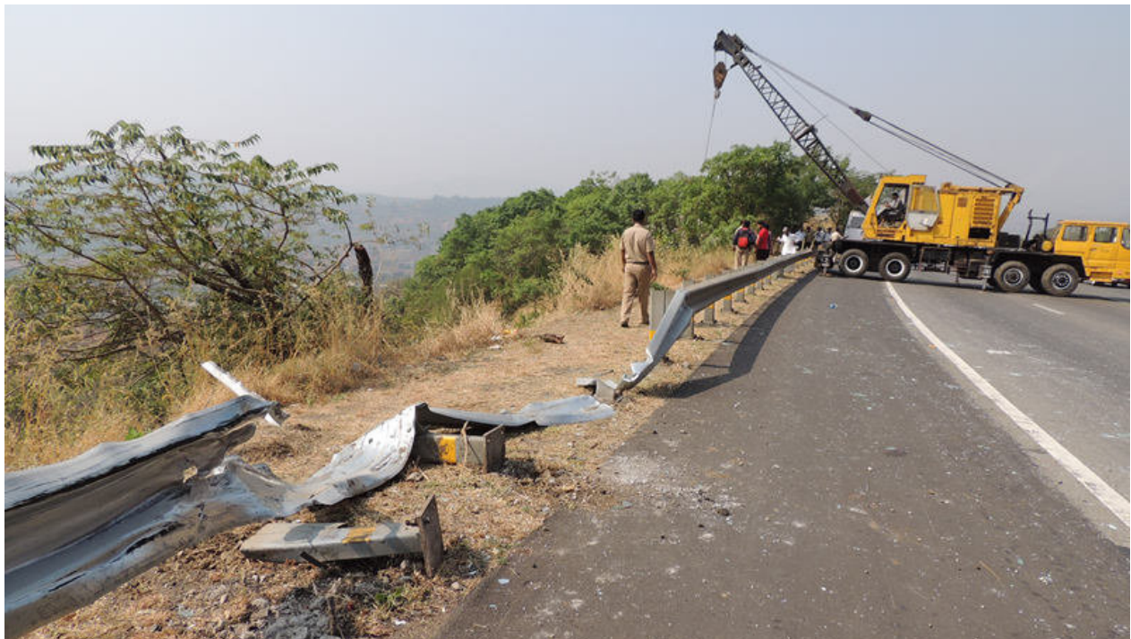
Figure 4. Cliffside barrier breached in a crash
