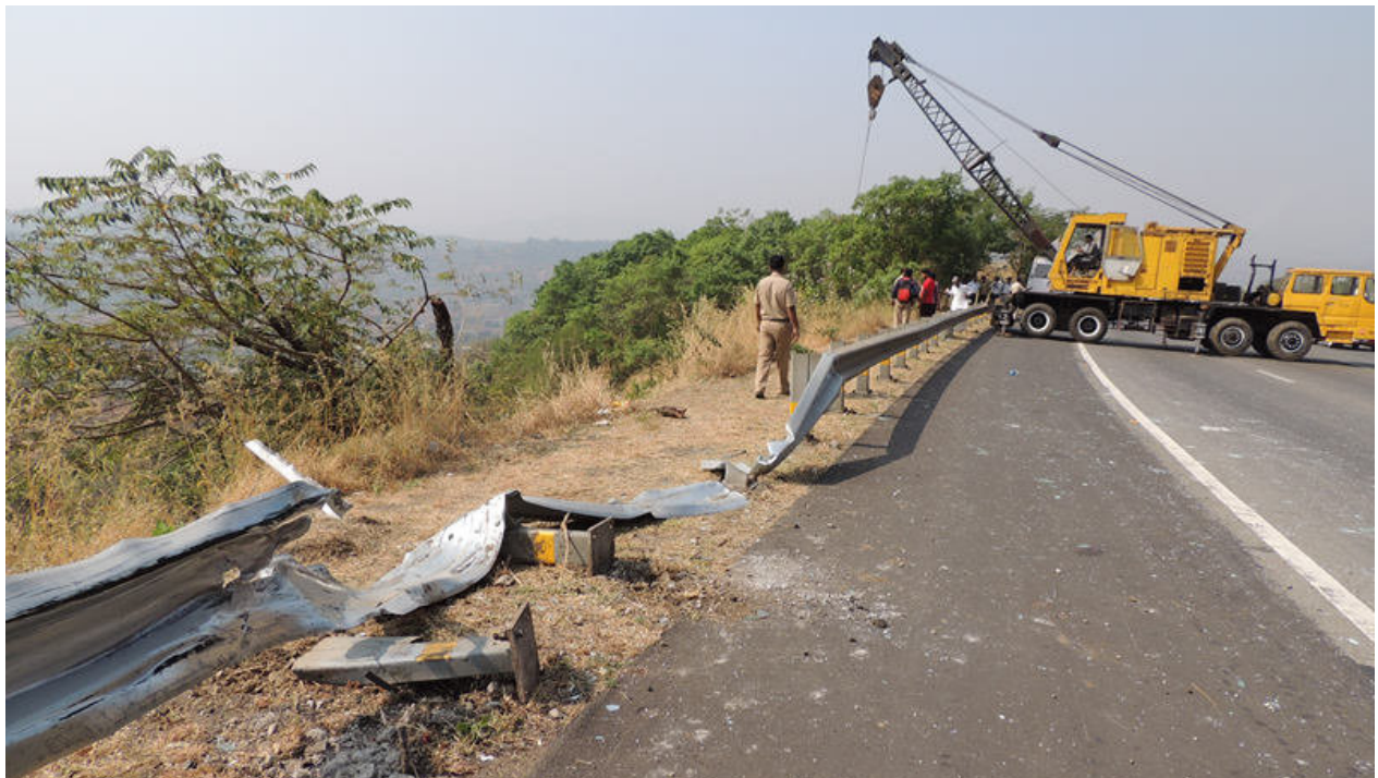
Figure 4. Cliffside barrier breached in a crash
